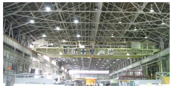
Inside the factory after the lighting changeover. LED lighting not only consumes less electricity, but its dimming control function helps control light levels, and it can be immediately turned on without any idling, which contributes to energy savings and electricity conservation.
